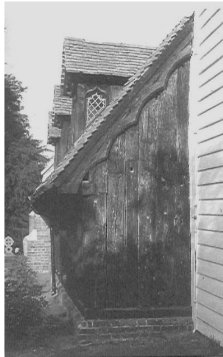
Probably the oldest standing timber building in the UK, dating from around 1000 AD, The Church of St. Andrew, Essex. Picture: Appraisal and Repair of Timber Structures
