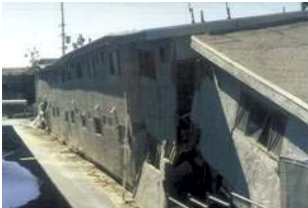
Figure 11: Failure of the Northridge Meadows apartment complex during the 1994 Northridge earthquake
