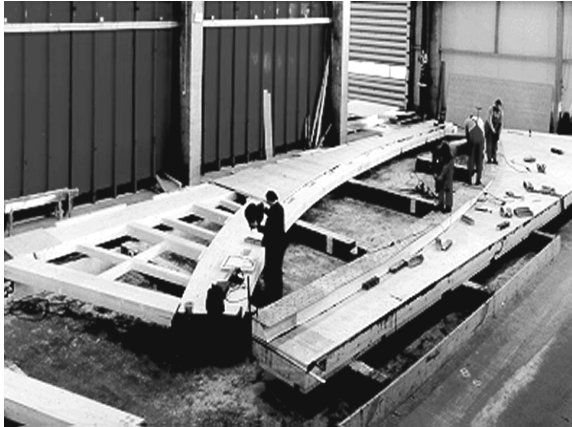
Figure 11. The assembly of the box-beams of girder. The flanges are made of glulam and two Kerto-LVL panels thickness of 33 mm are screw glued both sides of flanges. The upper flange is straight and the lower one is curved
