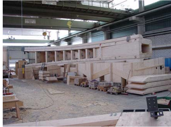
Figure 12. One cantilevered truss consists of two box beams, which are braced against lateral deformation. The weight of one element is 35 tons.
