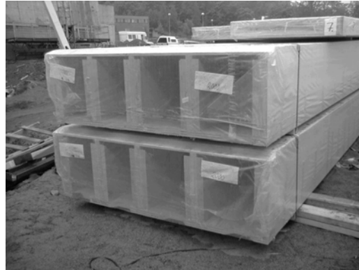
Figure 10. LVL stressed skin panels as balcony elements stored in the construction site.
