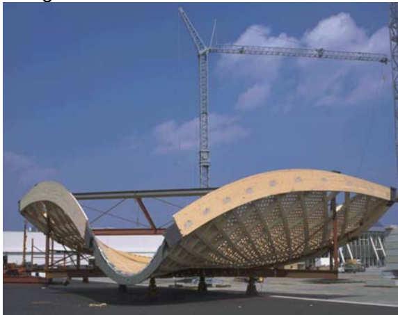
Figure 13. Double-curved lattice shells has been screw glued close the site in one of the exhibition halls Hanover.
