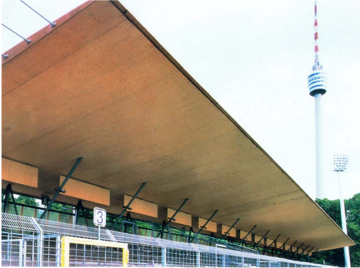
Figure 8. Light and airy roof construction gives wide view over the playing field. The roof consist of 15 elements 6.78 m wide and two 1.15 m wide elements in the both ends. The length is 104 m and area of 1,800 m 2 .
