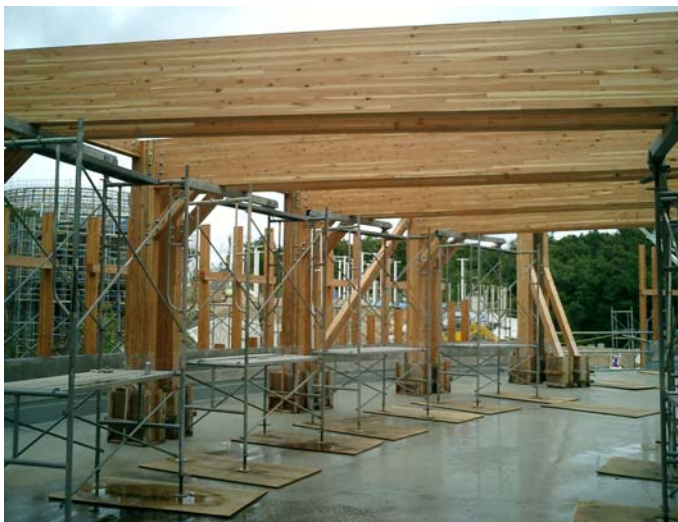
Illustration 27: Pergolas on the top floor (4 th floor=roof terrace), that would be easy to remove by own joint details
