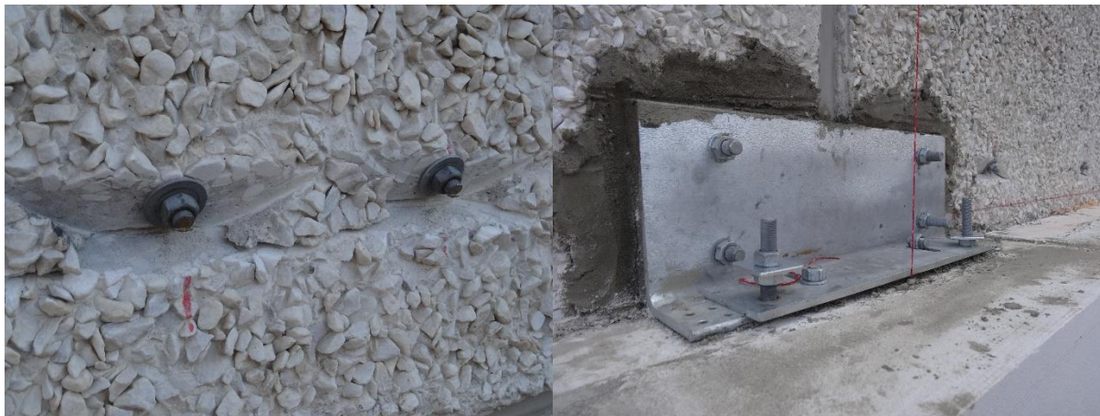
Figure 7: Original façade was strengthened with diagonal anchors (left). Modular wooden elements were hanged onto the existing wall surface with the help of designed fixings, allowing adjustment of modules in all three directions (right).
