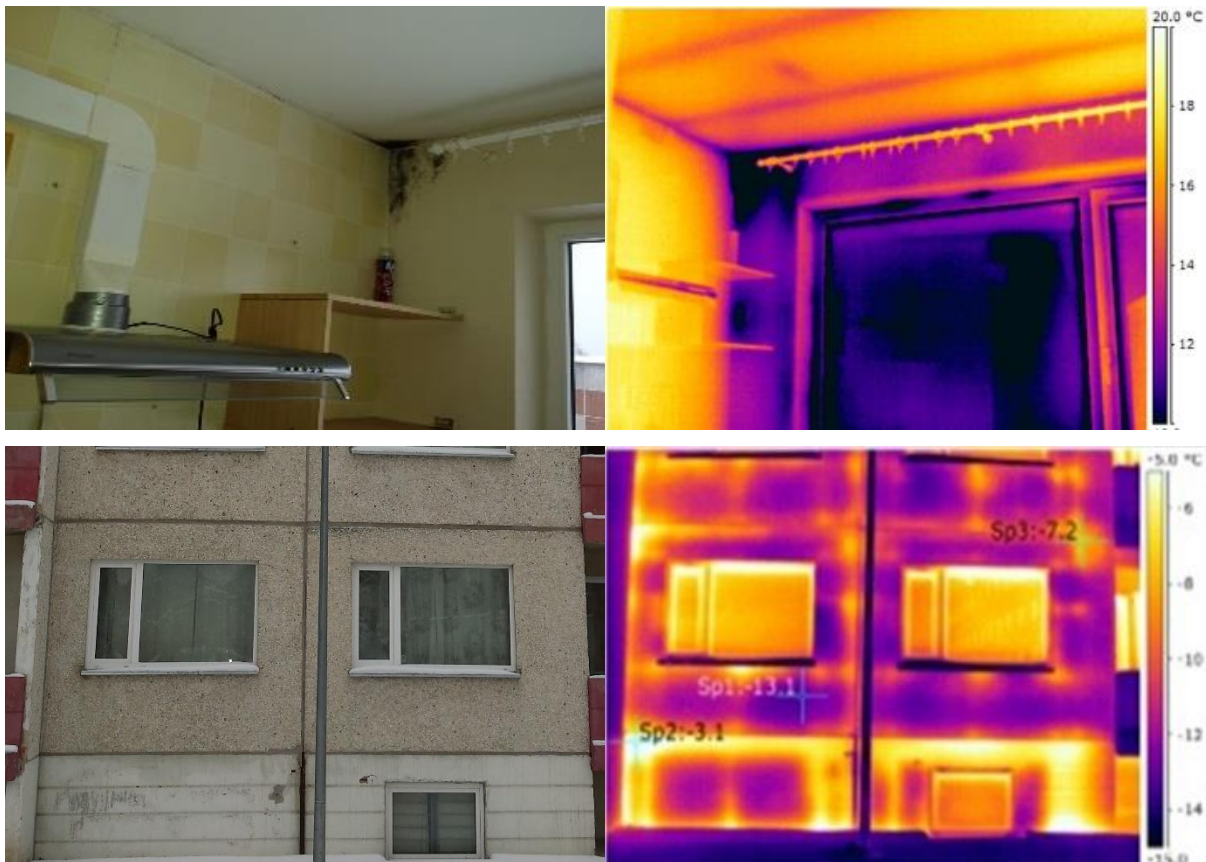
Figure 2: Overview of thermal bridges from inside (above) and outside (below) the building.
