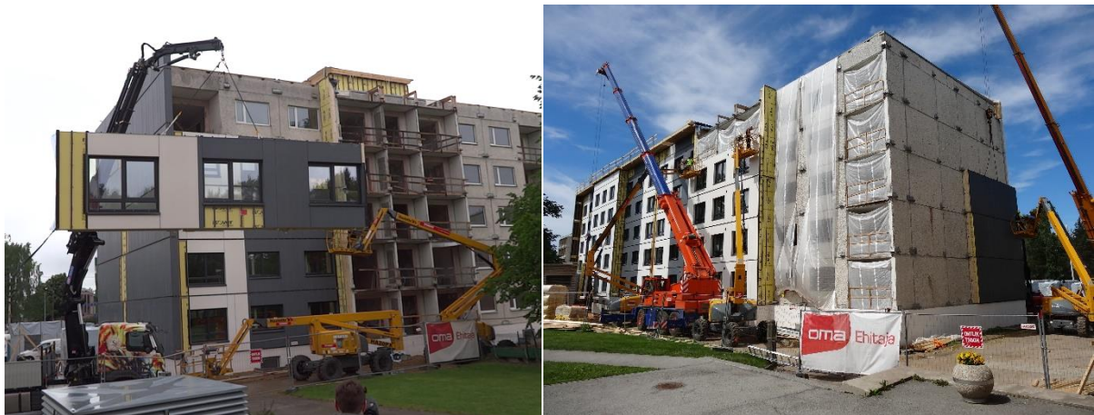
Figure 6: Wooden elements were mounted directly from a truck on two different façades at the same time. To minimize the influence of driving rain, façades were covered when waiting to mount panels.
