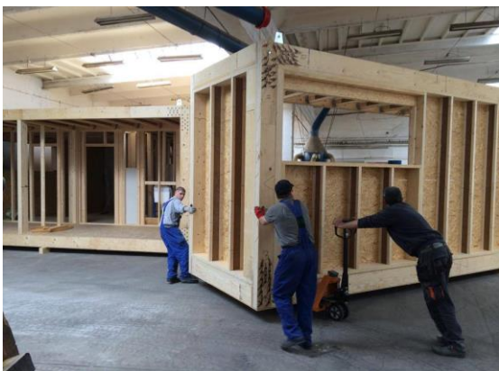
I-joists: as wall studs by modular houses production process. Photo: Rebel Module
