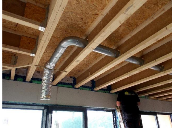
I-joists: service holes made in the middle of the web. Photo: Szreder A.C.
