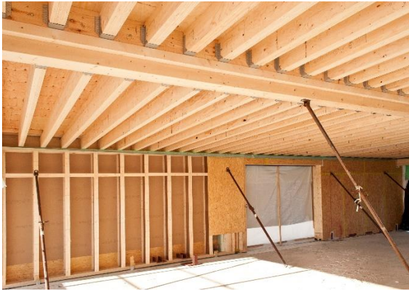
LVL R: secondary beams in floor construction. Photo: STEICO
