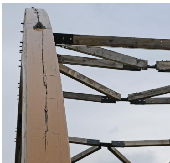
Figure 6: Arches are uncovered. Some cracks discovered on the upper side.
