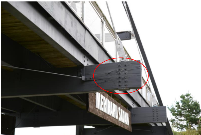
Fungal damage of the transversal beam
