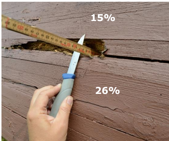
Moisture contents measured above and below the crack.
