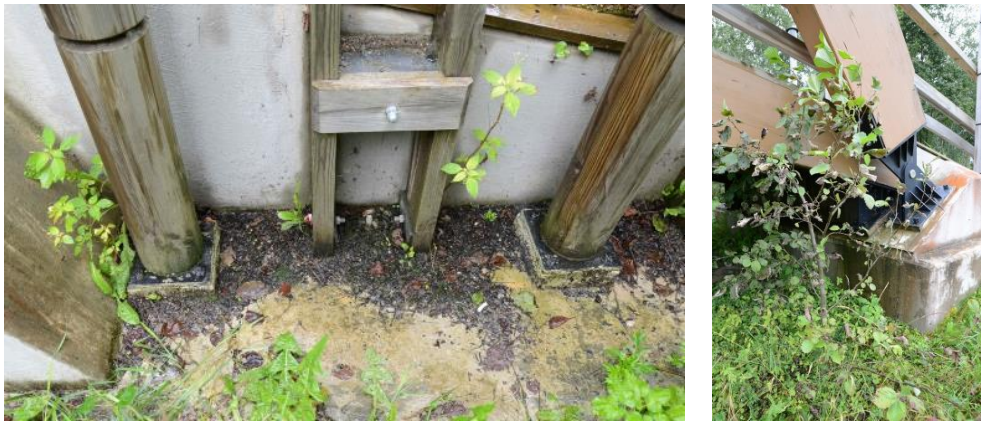
Figure 7: Dirt and gravel on all parts of the substructure due to lack of preventative maintenance.
