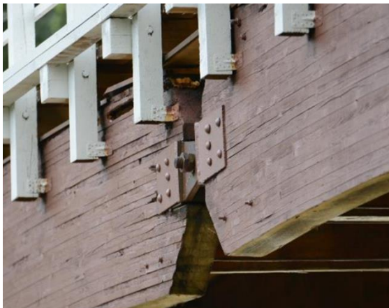
Deformation and decay in the top of the arch, the hinge is lost.
