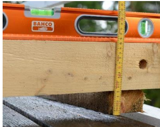
Bridge deck tilted 52mm /m, due to local failure in the arches connection points.
