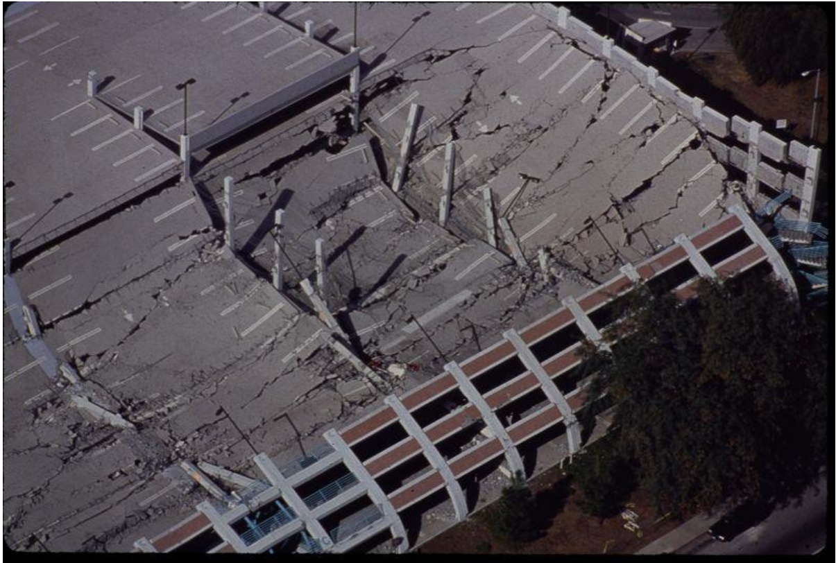
Figure 2: Collapsed parking structure at California State University Northridge, 1994 Northridge earthquake. While extremely ductile concrete moment frames around the outside formed the vertical elements of the LFRS, the interior gravity support structure was not detailed for displacement compatibility to accommodate the interstory drifts permitted by the moment frames, leading to collapse of the structure even though the vertical elements of the LFRS were very good. (Source: EERI)
