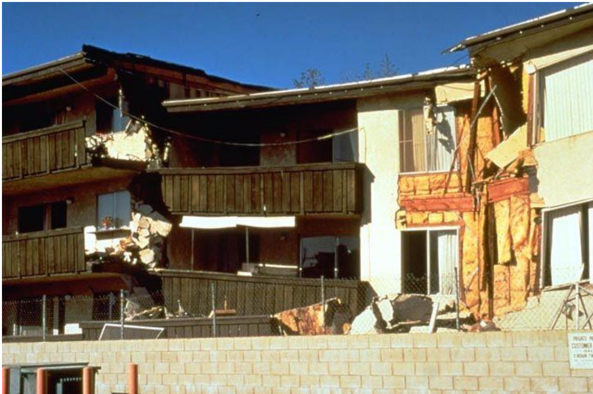
Figure 1: The Northridge Meadows apartment complex where sixteen residents died in the 1994 Northridge earthquake of southern California. The collapsed first story contained a mixture of living spaces and parking units. (Source: EERI)
