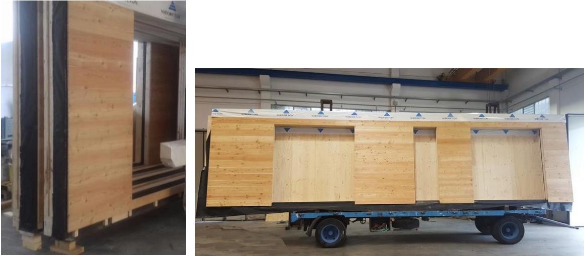
Figure 4+5: Prefabrication of the wall in the factory with cladding and transport to the building site.
