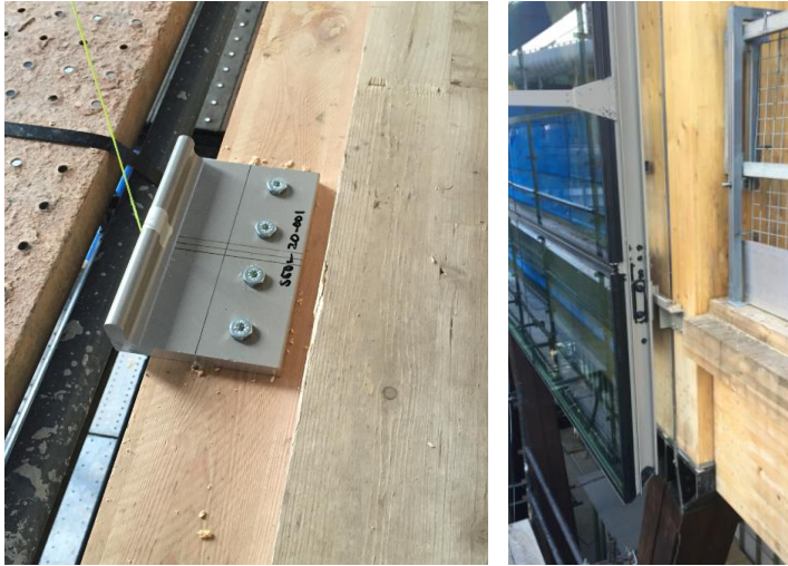
Figure 10: Façade slab edge bracket (left), column bracket and first façade panel installed (right)
