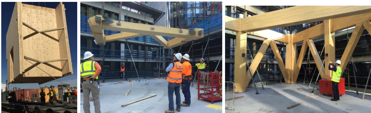
Figure 11: Pre-assembled lift core (left), braced bay lifting (middle), and installed braced bay (right)
